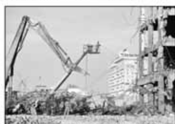
Building Trades members take part in the demolition of the historic Ambassador Hotel, built in 1921.
